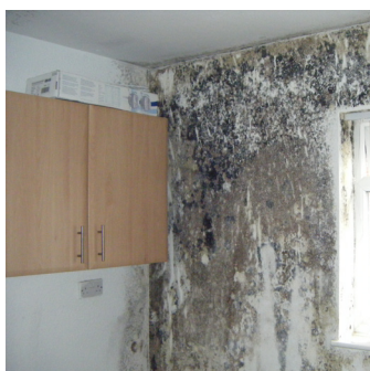
3 Mould growth to the externl kitchen wall
