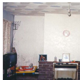
5 Mould growth to the living room wall
