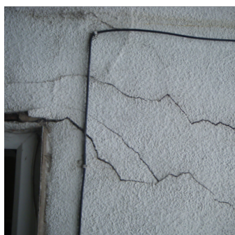
2 External wall with cracks to rendering
