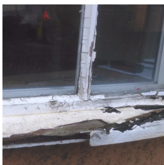
4 Condition of the wood to the windows
