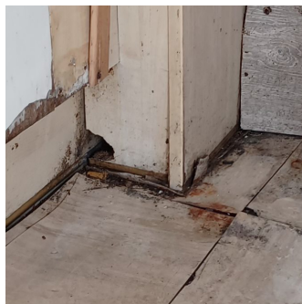
3 Poor condition of kitchen floor tiles
