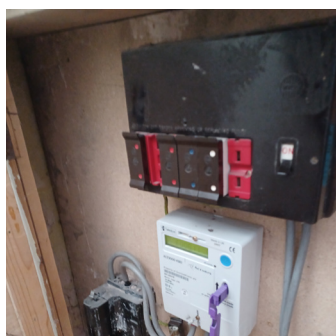
2 Consumer unit to understairs cupboard
