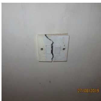
3 Cracked light switch to kitchen
