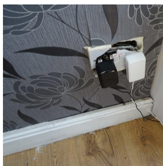
4 Broken socket to living room
