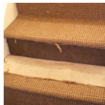
4 Loose carpet on staircase
