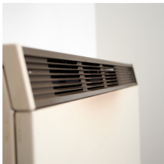
5 Storage heater in front bedroom
