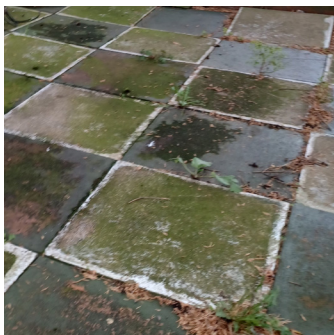
4 Front yard uneven slabs
