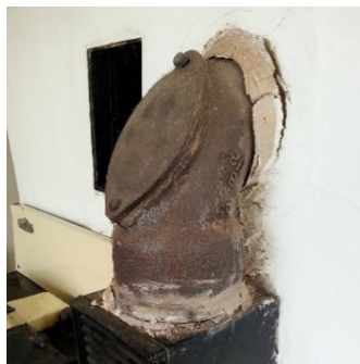
4 Cracked clay around base of flue
