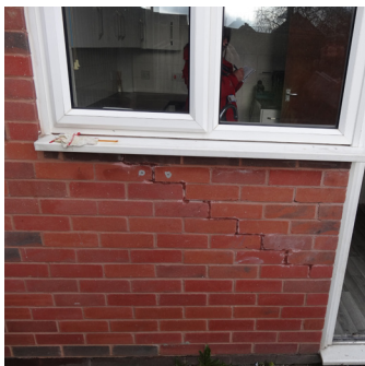
2 Crack below the kitchen window
