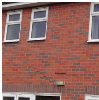
4 Crack above the kitchen window
