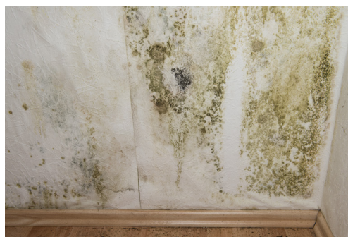
4 Mould growth to the small rear bedroom
