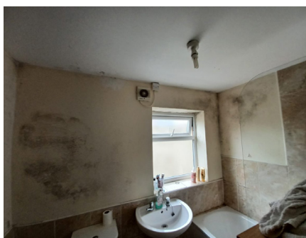
3 Mould growth to the bathroom
