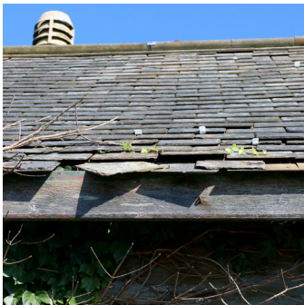
3 Roof with slipped and missing slates
