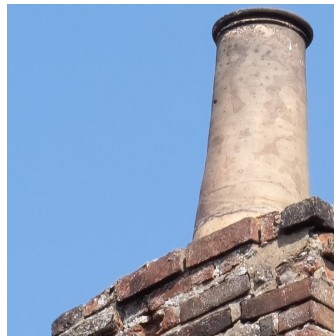
5 Disrepair to chimney
