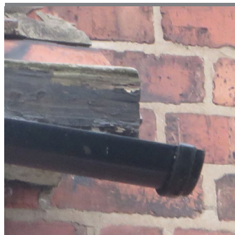
4 Loose rear eaves gutter
