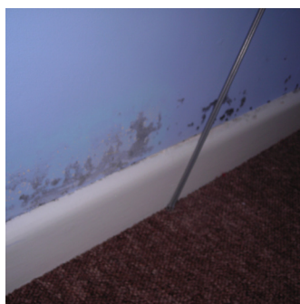
5 Mould growth in smallest bedroom
