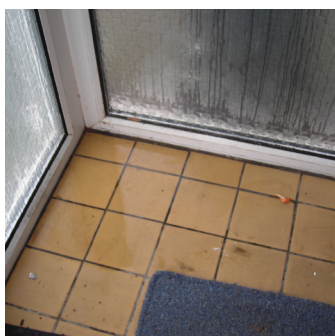
4 Pooling water on porch floor interior
