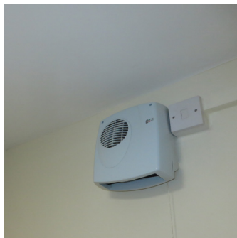
4 Fan heater in the bathroom
