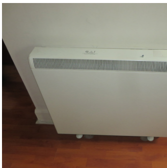
3 Storage heater in the bedsitting room
