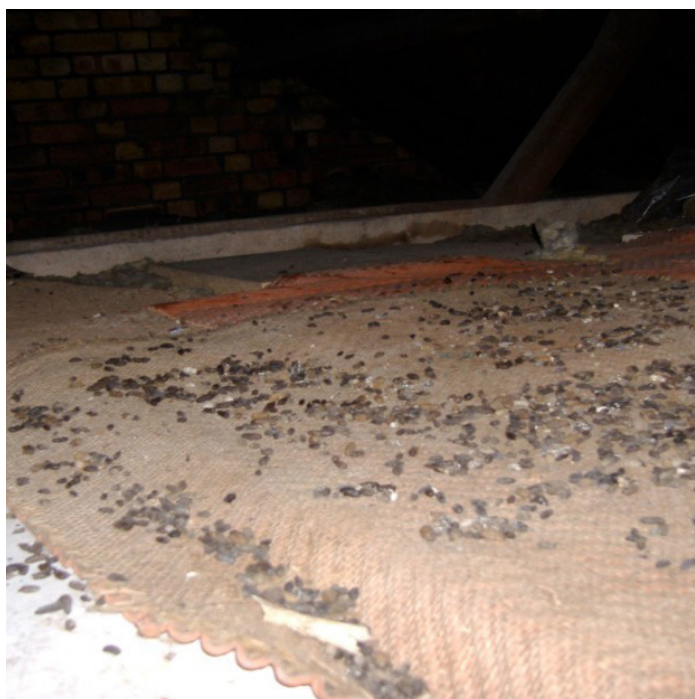
4 Droppings in loft space
