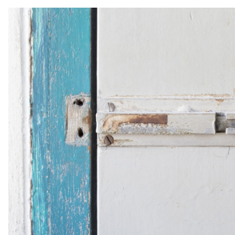
8 Broken bolt to bathroom door
