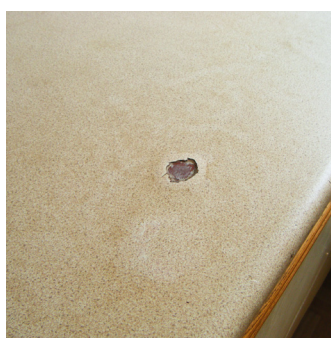
7 Close-up of damage to kitchen work surface
