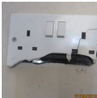
4 Broken socket in living room
