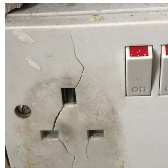
5 Broken socket in living room
