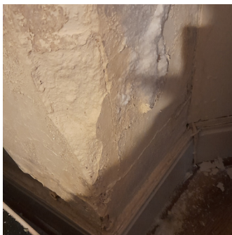
5 Damp salted internal plaster
